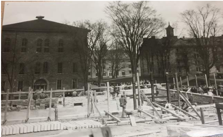
Figure 1: This is a photograph of the construction of Stillman Hall in 1927. It highlights the tidy and well-kempt construction site (Untitled photograph of Stillman construction, 1926).
