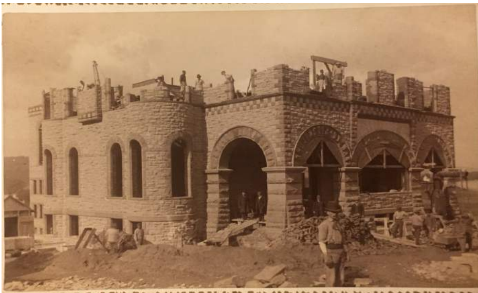
Figure 6: This is an image of the construction of James B. Colgate Hall. This image also highlights the stone and locally made brick utilized on the exterior of the building ([Untitled photograph of James B. Colgate Hall], A1000 Box 10 Folder 10)
